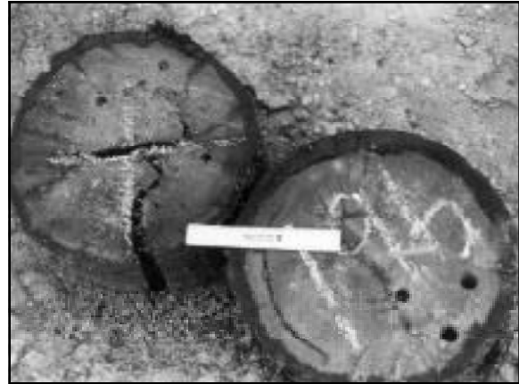
When the first salvaged piling failed, a second was driven, which also failed. Note marine borer damage in both.
