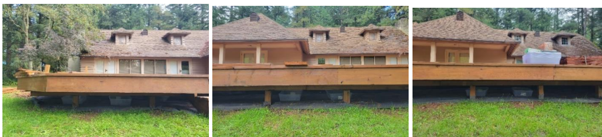
Figure 1: Photo of the CA-C treated deck with three sampling locations and six sampling basis underneath the front of the deck.
