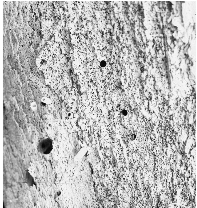
Figure 1.8 Wood damaged by Limnoria showing tiny tunnels on the wood surface along with larger tunnels left over from shipworms.
