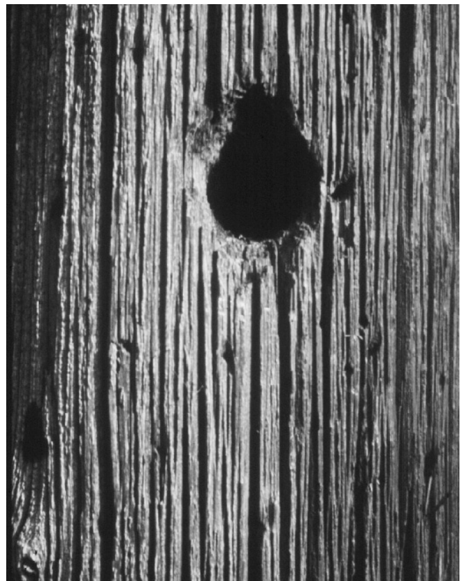
Figure 1.9 Woodpecker cavity in a utility pole. These holes allow water, fungi, and insects to enter the wood, accelerating deterioration.
