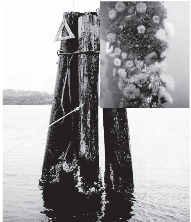
Figure 9.13 Sooke Basin dolphins constructed in support of Environment Canada's creosote evaluation study.
