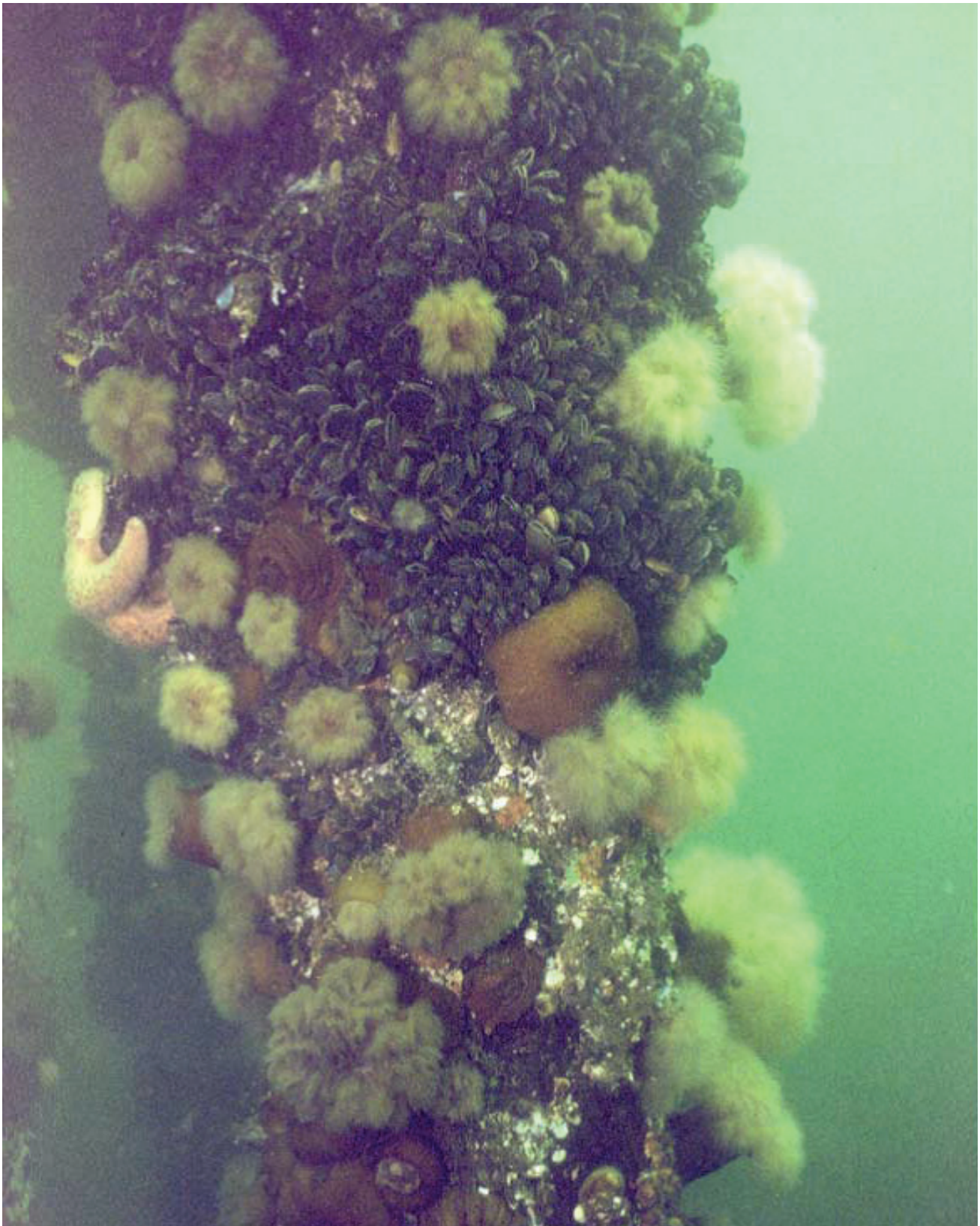
Figure P2. Creosote piling treated using BMP procedures and exposed for two years in the Sooke Basin. Barnacles dominated at the highest intertidal elevations, but were displaced by mussels, which also would have invaded deeper elevations were it not for starfish and crab predation. Several species of anemones proliferated below the mussel zone.
