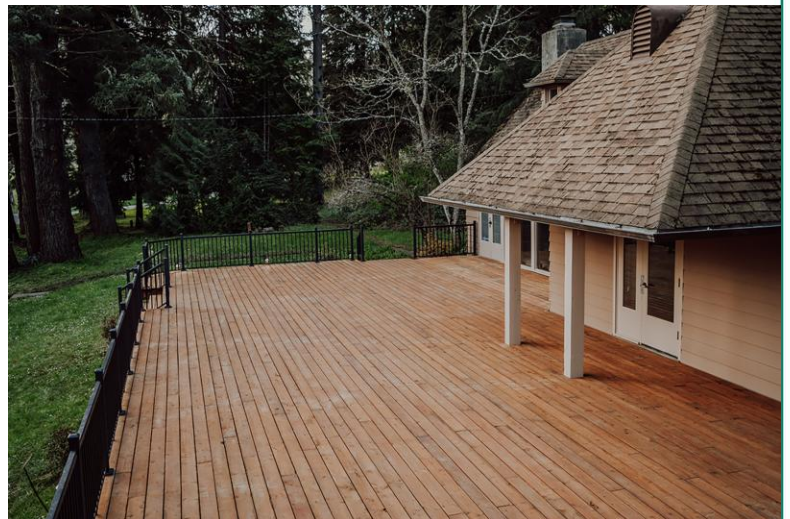
The deck at Oregon State University's historic Peavy Lodge, where researchers confirmed the preservatives in today's preserved wood do not leach from the wood and contaminate soil or rainwater runoff.
