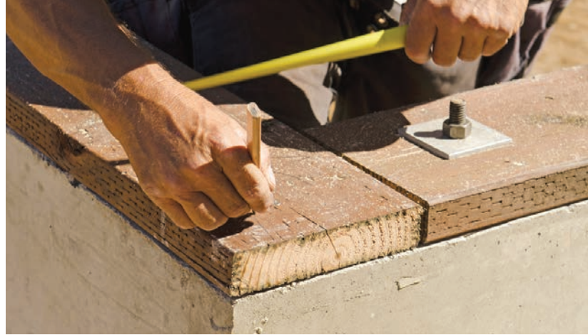
Pressure-preservative-treated wood used as sill plates. The IBC requires that surface treatments be applied to end cuts and holes.
